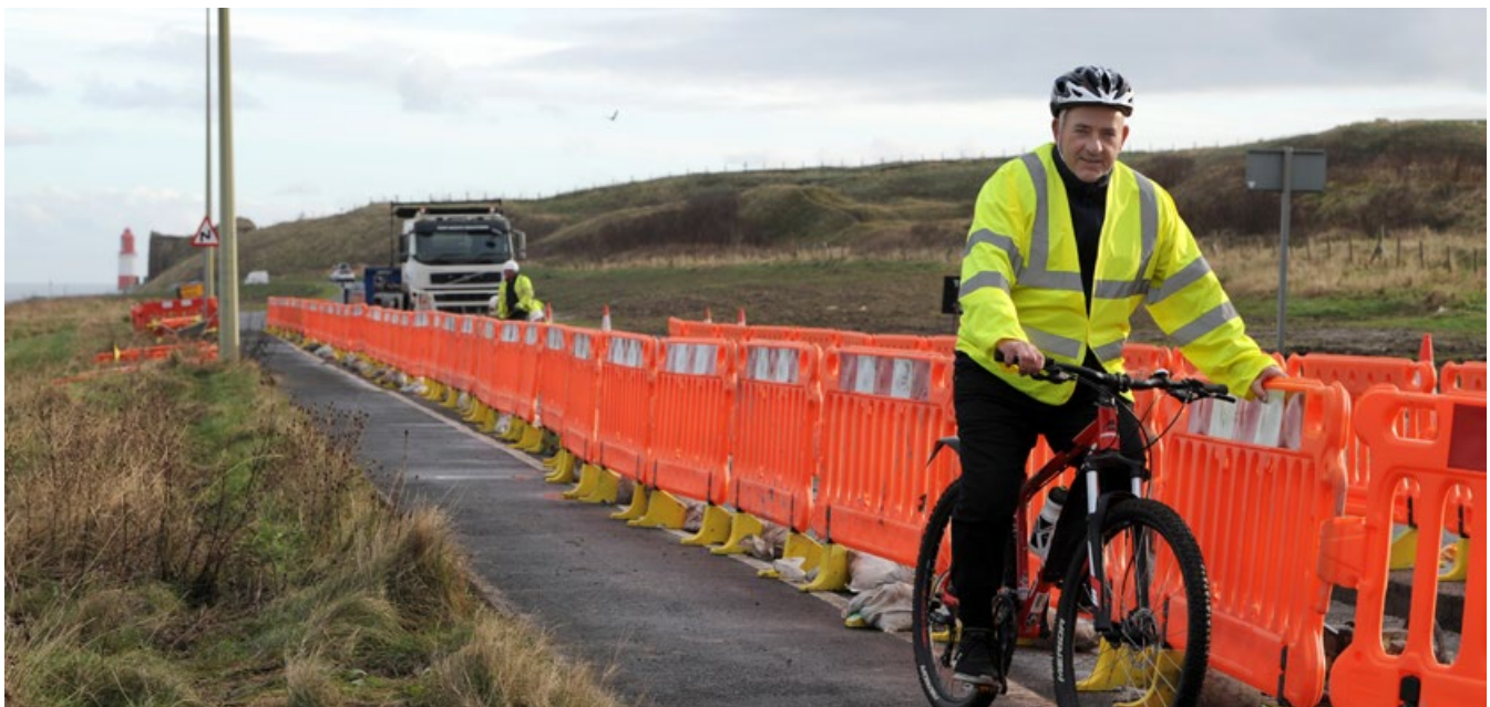
CLlr Gibson at the Coast Road Alignment project which was shortlisted for 'Project of the Year' in the Chartered Institute of Highways and Transports North East and Cumbria Awards
