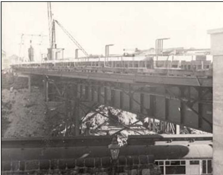
1937: River Drive Bridge under construction (photo courtesy of South Tyneside Libraries & Information).
