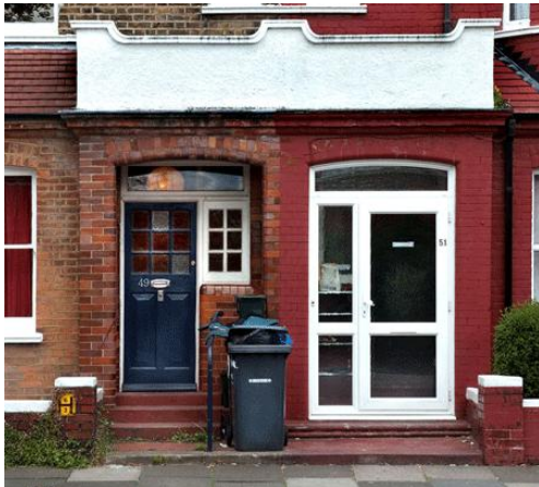
The above image clearly shows how the use of inappropriate materials and detailing can have a detrimental impact on the character and appearance of a property.
