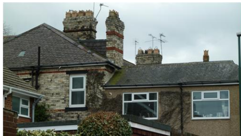
The extension to the rear of the period property above is at odds with the character and appearance of the original building, largely due to scale and choice of materials.
