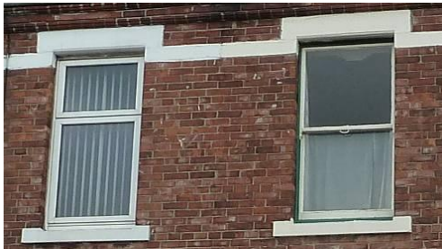
The timber sash window on the right (above) retains its elegant proportions and appearance, whilst the uPVC window on the left is bulky in comparison.
