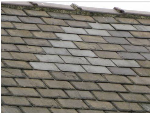
A roof at Mariners' Cottages has been repaired using appropriate matching materials that blend in well with the roofline. These newer materials will weather over time.
