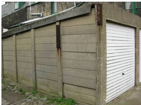
Many alterations and additions, such as the garages above, were erected before the Cottages were Listed. The Management Plan will help ensure that any future alterations are more in keeping with the character and appearance of the Conservation Area.
