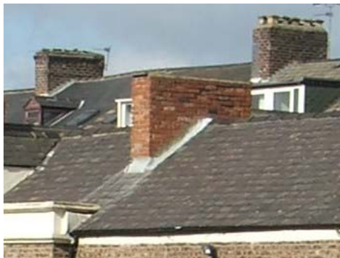
Over a long period of time many alterations have been made to the chimneystacks at Mariners' Cottages. Some have been reduced in height, pots have been lost, and television aerials have been installed, which can be quite damaging to these structures, not to mention unsightly. This is a common problem throughout all Conservation Areas.
