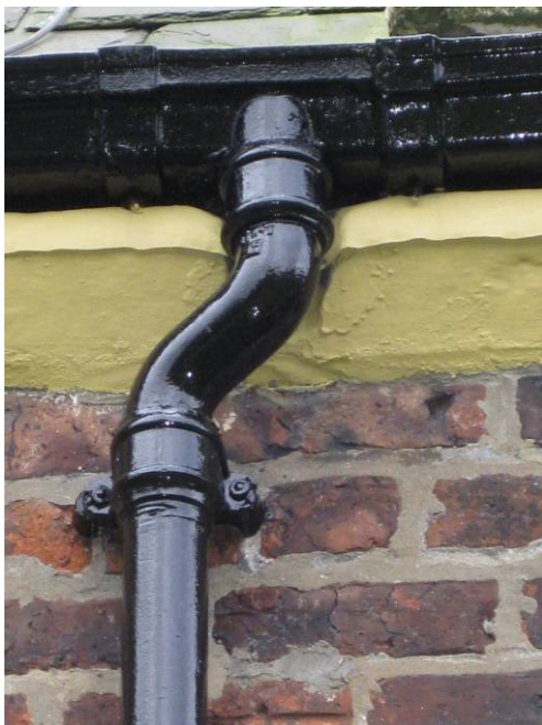
The original cast iron rainwater goods have been repaired and repainted as part of Grainger Plc's recent improvement works.
