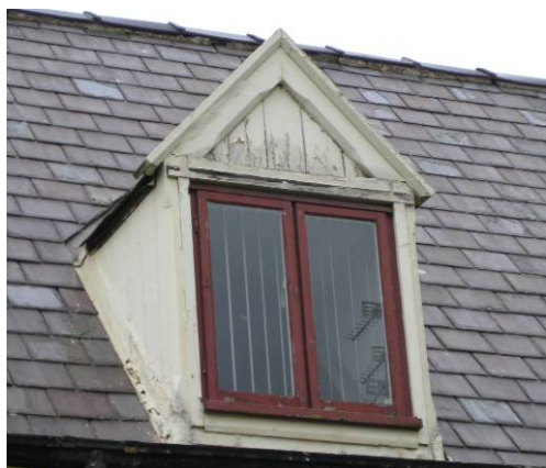
Years of neglect by previous owners left the dormers beyond repair.
