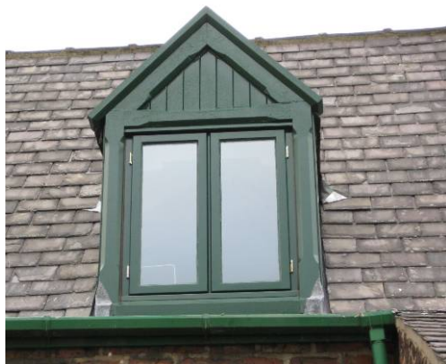
Since taking ownership of the Cottages, Grainger plc is well on their way to replacing all the defective timber dormer windows to their original design throughout the eastern terrace of Mariners' Cottages. Regular maintenance should see these windows lasting for many decades.
