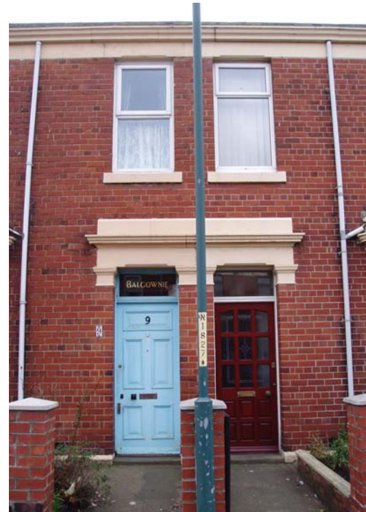
Figure 44 Terrace house detailing (showing original door on left and modern replacement on right). Windows are modern upvc replacement and original cast iron downpipes replaced with plastic.
