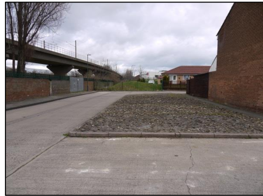
Photograph 4: Area of initial ponding of surface water
