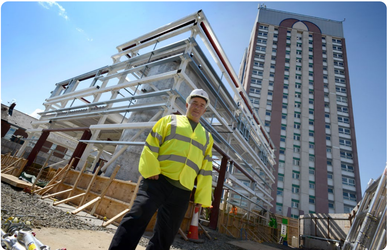
Cllr Ernest Gibson visits the site of the Hebburn Renewable Energy Scheme
