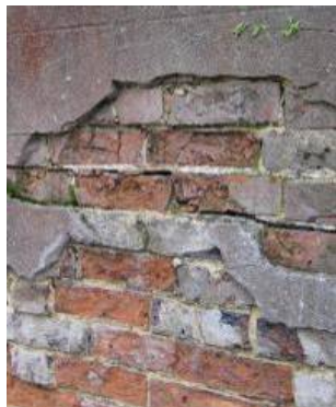
This cement render has failed, leaving behind brickwork that has been damaged as a result of the impermeable render trapping water inside the wall (freeze-thaw action). A lime render would have allowed the water to harmlessly evaporate.
