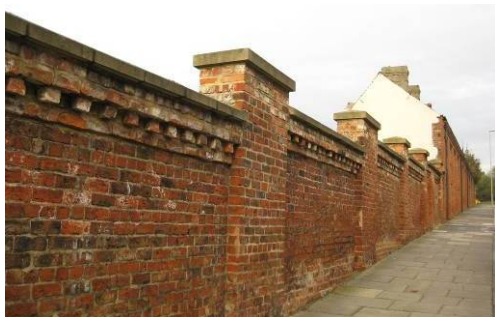
Staithe House and the adjoining wall are key elements of the streetscene.
