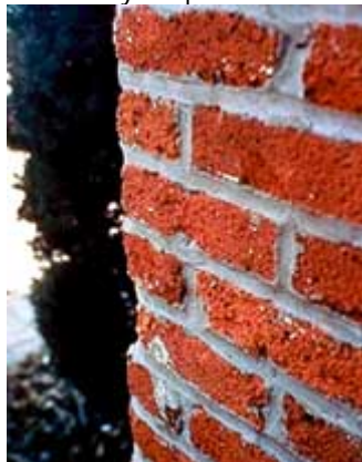
Abrasive cleaning causes permanent damage to brickwork. This has been compounded by the use of inappropriate cement mortar and poor quality re-pointing.
