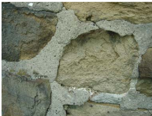
This wall has been re-pointed using a cement-based mortar. The softer stonework has eroded, leaving behind the hard mortar.
