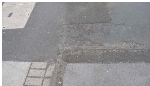
Repairs carried out by utility companies along Front Street have left an unsightly patchwork of materials.
