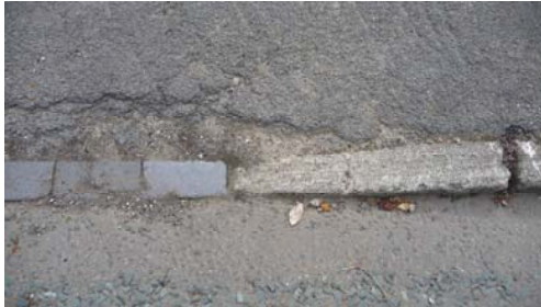
Natural stone kerbs and traditional scoria blocks can be found along Underhill Road. Such features should be retained.
