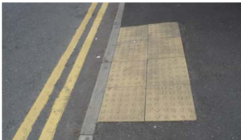
Buff tactile paving and standard yellow lines can detract from the character and appearance of Cleadon Conservation Area.
