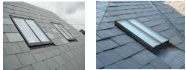
The conservation style rooflights on the left lie flush with the roof, whilst the standard rooflights on the right are more obtrusive.
